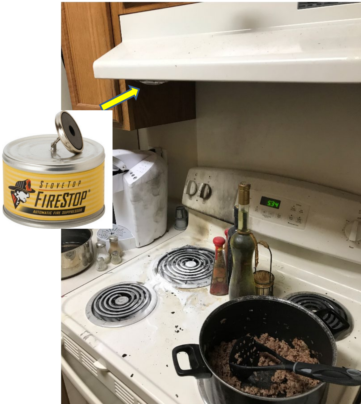
CUTLINE: This photograph shows a StoveTop FireStop device in place above the range top. The device over the fire activated and extinguished the flame.
